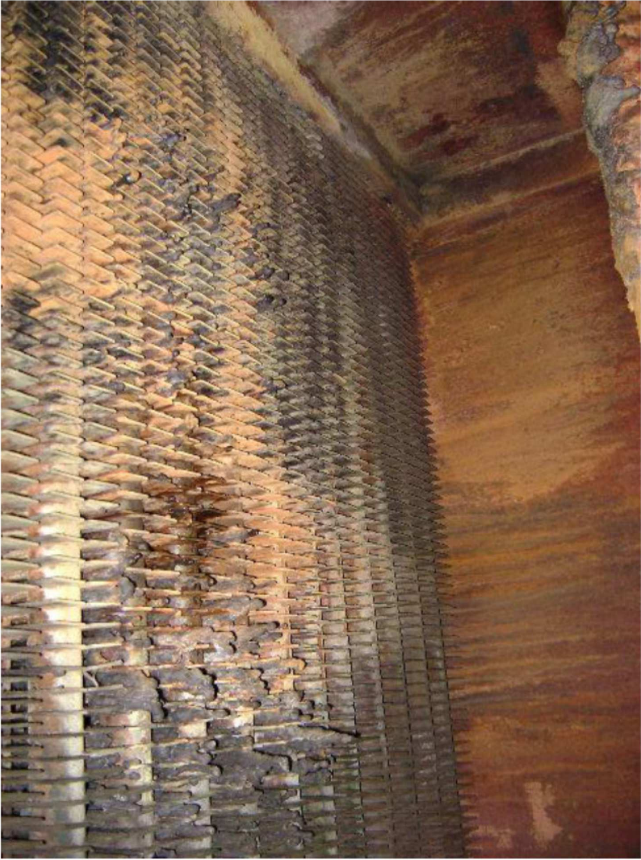
Lower side of middle evaporator tubes section with melted metal.
