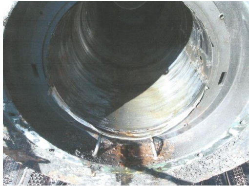
Fig. 1. Condition of aft and fore of stern tube bearing
